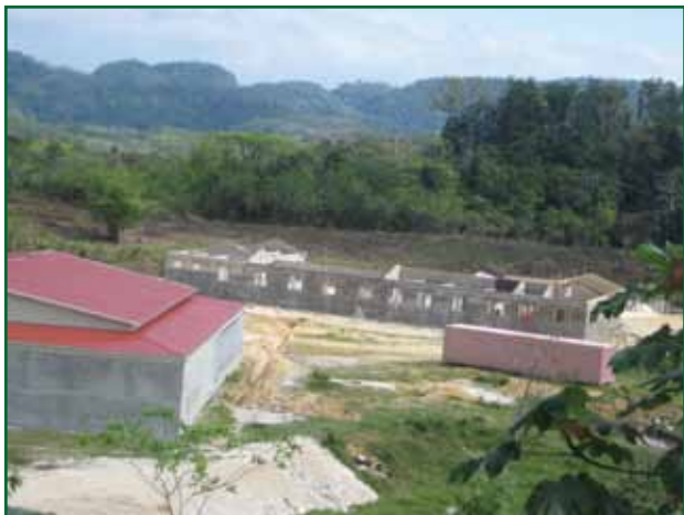
The construction of the Sisters' new clinic and the parish sausage factory at the Jamaican mission.
